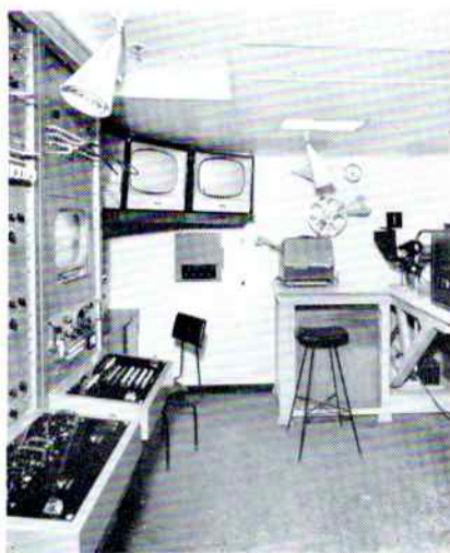
TELEVISION CONTROL ROOM
