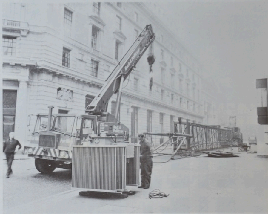
▲ While workmen prepare the transformer for the 'big lift' the crane is assembled.
