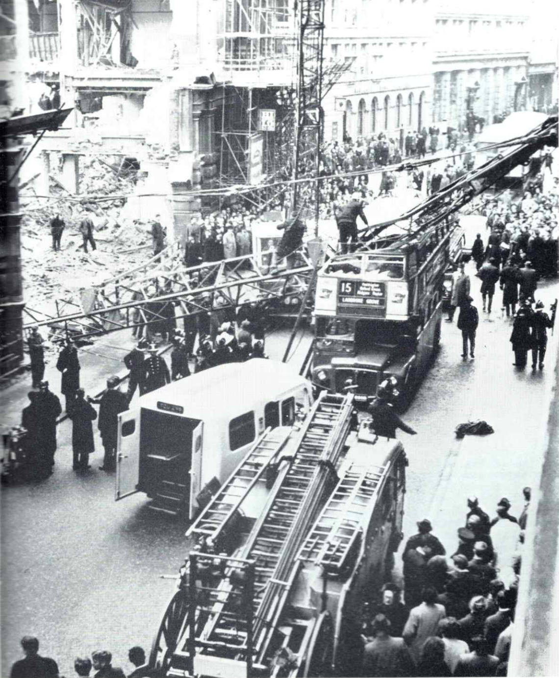
'122' Still in the News. It had become a melancholy pastime, especially in the lunch hour, to gaze on the rapidly lessening structure of our old offices. Then one day, April 3rd, the old address appeared again in the evening papers, when a crane arm collapsed and fell across Leadenhall Street. The driver of an approaching omnibus saw it as he was approaching but could not avoid the mishap. The crane fell right across the bus injuring a number of passengers in the top deck but fortunately none was seriously hurt.
