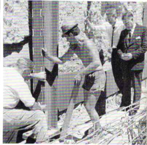
Mr. N. D. Pixley (right), Chairman of P & O-Orient Lines of Australia Pty. Limited, watches the first column of the new P & O Building in Sydney being placed in position. The building, scheduled for completion late in 1963, will rise to 18 floors.
